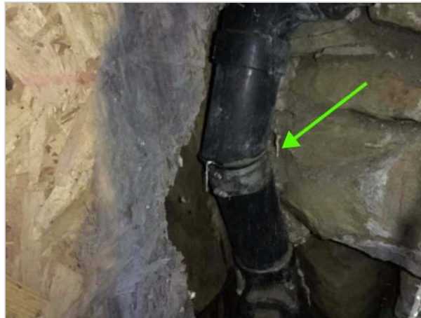
Drain stack pushed by foundation.
