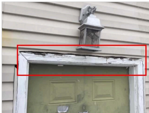
Rotted wood example.
