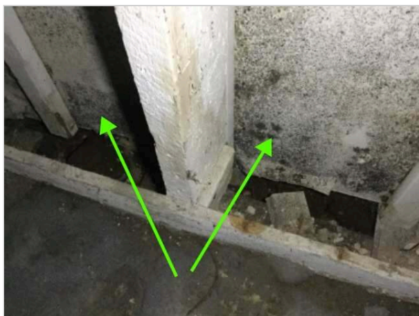
Basement mold like substance example.
