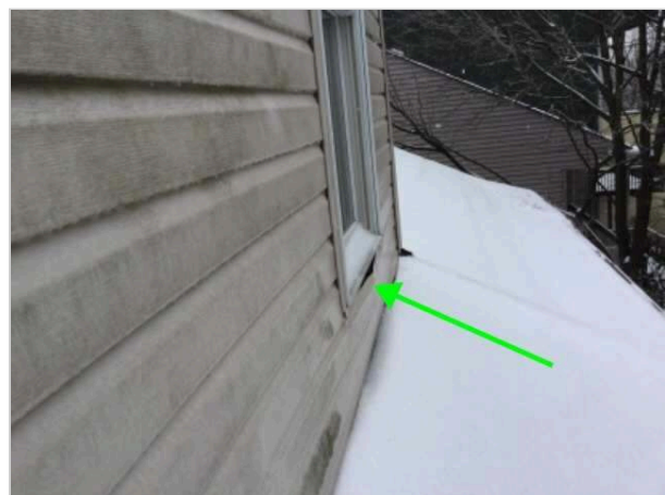
Loose siding on back
