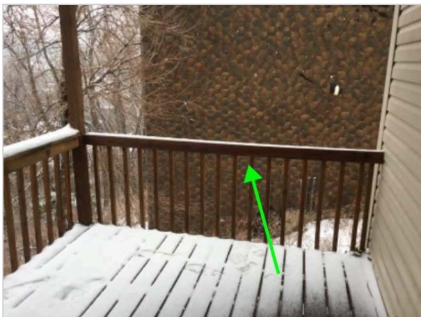
Loose deck rail
