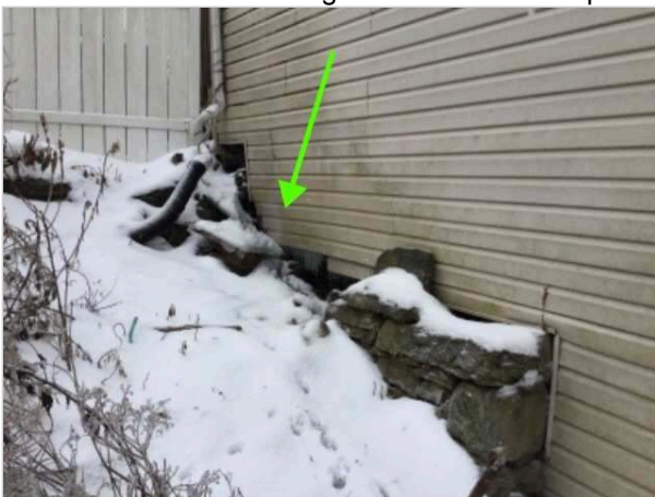
Front right foundation bowed inward.
