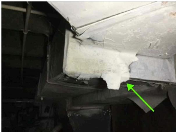
Possible asbestos material on ductwork.
