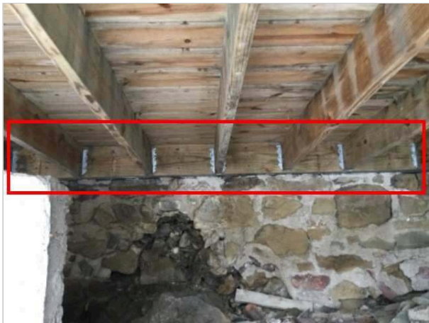
Deck ledger not bolted.
