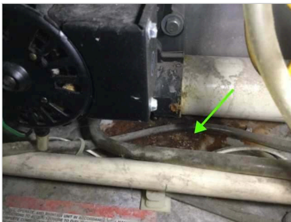
Evidence of previous leaks.
