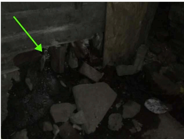
Water intrusion- right front.
