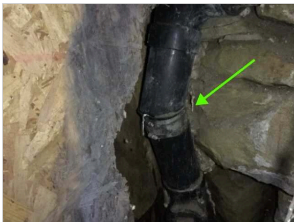
Drain stack pushed by foundation.
