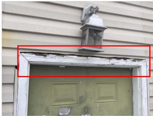
Rotted wood example.
