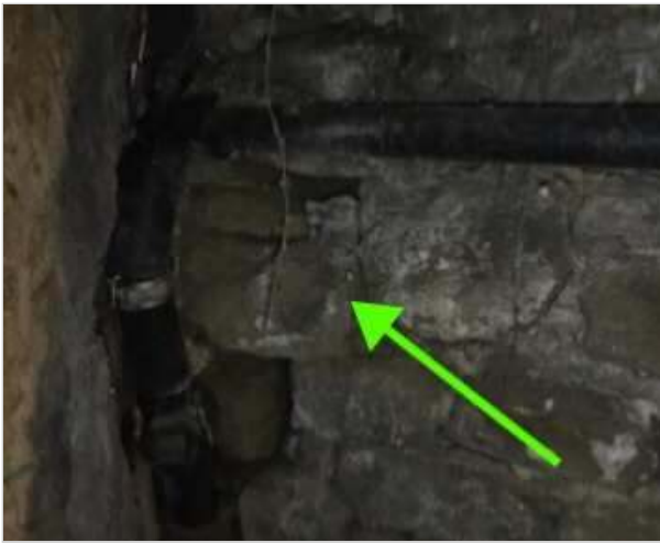
Front foundation wall in general state of disrepair.
