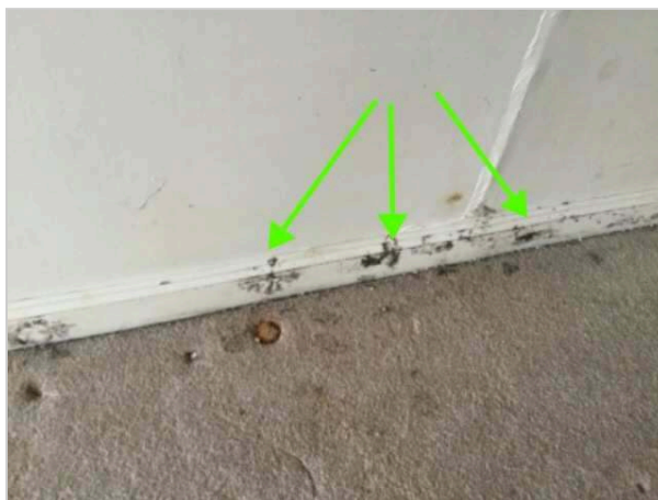
Mold like substance basement
