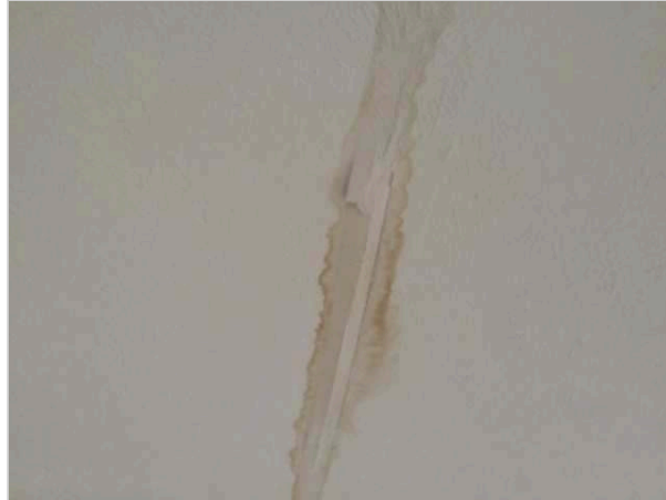
Watermark from previous leak
