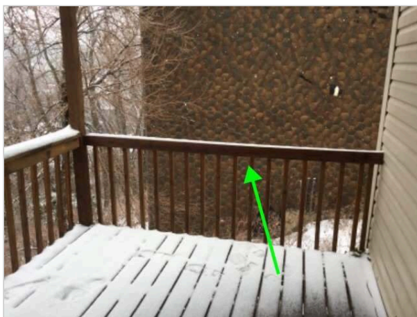
Loose deck rail
