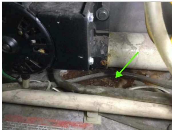
Evidence of previous leaks.
