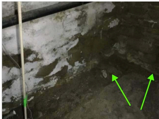
Basement moisture left front
