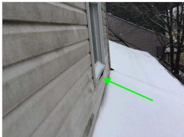
Loose siding on back
