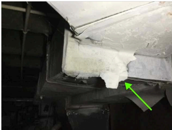
Possible asbestos material on ductwork.
