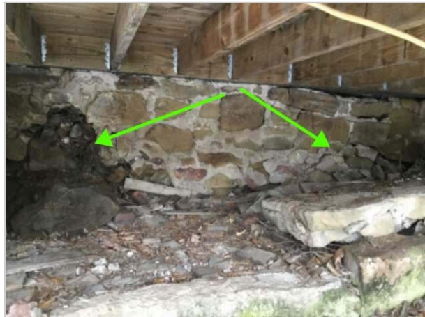
Rear foundation wall in general state of disrepair.
