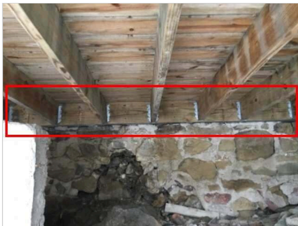
Deck ledger not bolted.
