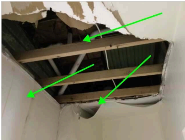
Ceiling and wall damage from pipes leaking
